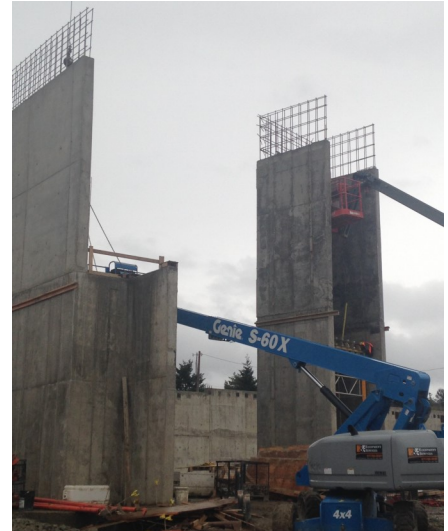
Below: Overview of the progress of concrete slab along the east edge of the building and shear walls for the upper level. Right: Elevator shaft.
