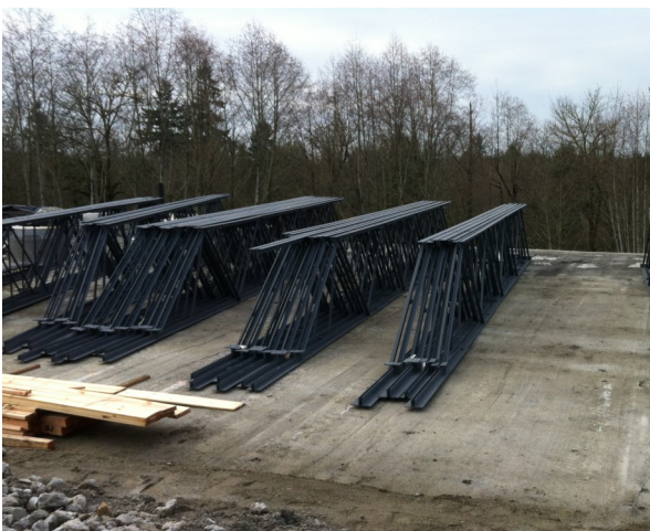
Steel stored on top of the vault.
