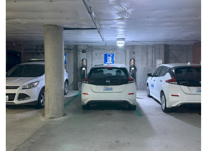
Figure 6. EV charging at Sammamish City Hall
